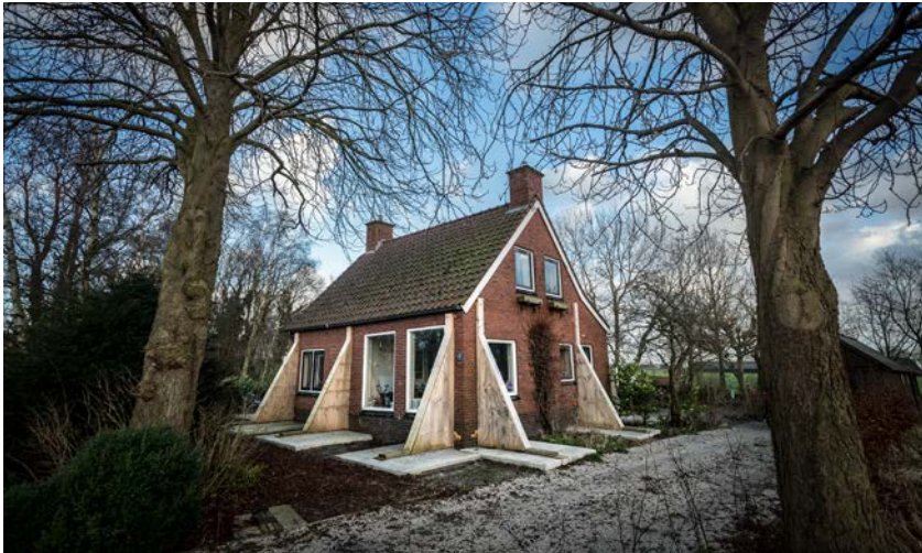
Figure 2: Damages caused by earthquakes on a farmhouse in Lageland, 20 kilometres from Delfzijl. Source: Kees van de Veen.
